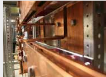
Busbars, LV boards
